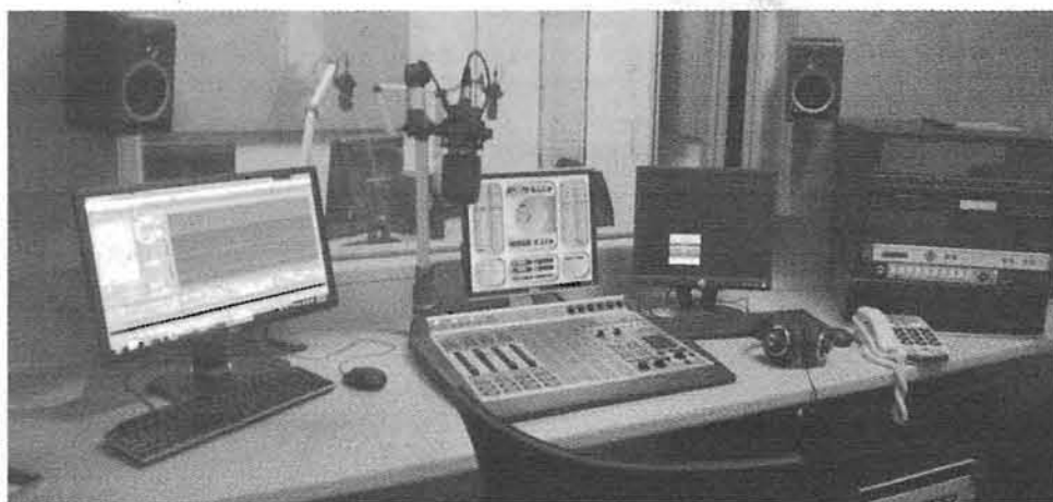
Control room at St. Louis Public Radio's new home Photo: Yeseul Park/The Current
